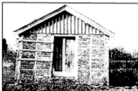
Rednal Warehouse, Montgomery Canal, showing the extent of leaning and settlement prior to work taking place
