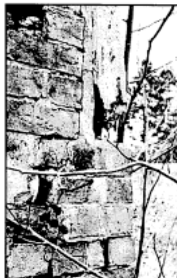
Example of building deterioration
